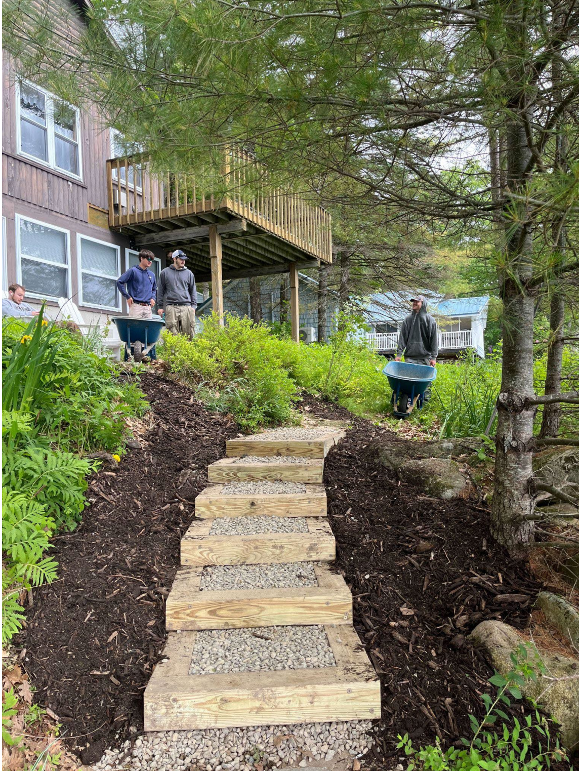
Left: Youth Conservation Corp crew member with a load of riprap for a shoreline stabilization project. Right: Completed YCC project on East Pond
